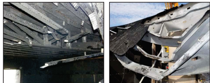
Figure 9, left: Gusset plate connection failure. Figure 10, right: Light-gauge steel C-joist warping.
