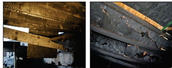
Figure 7, left: Dimensional lumber joist rupture. Figure 8, right: Web burn-through and subfloor separation.
